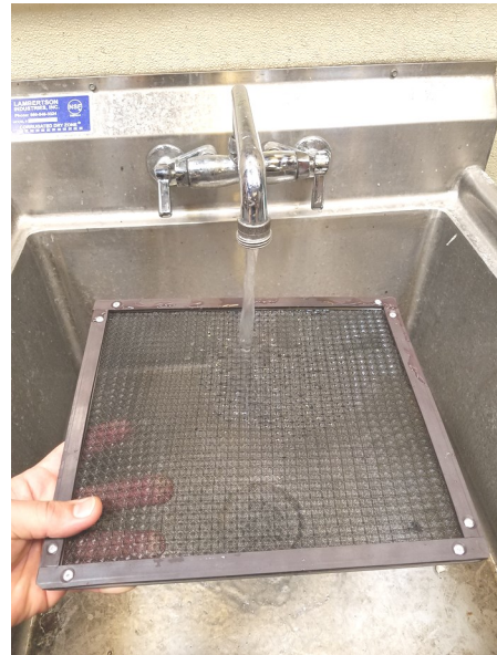
Condenser Filter Cleaning
